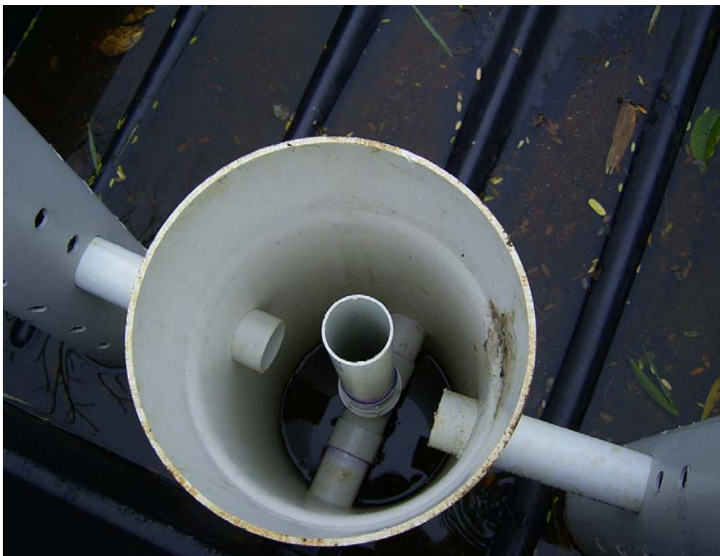
Plate 6. Water height adjuster inside a 300mm outlet tower
